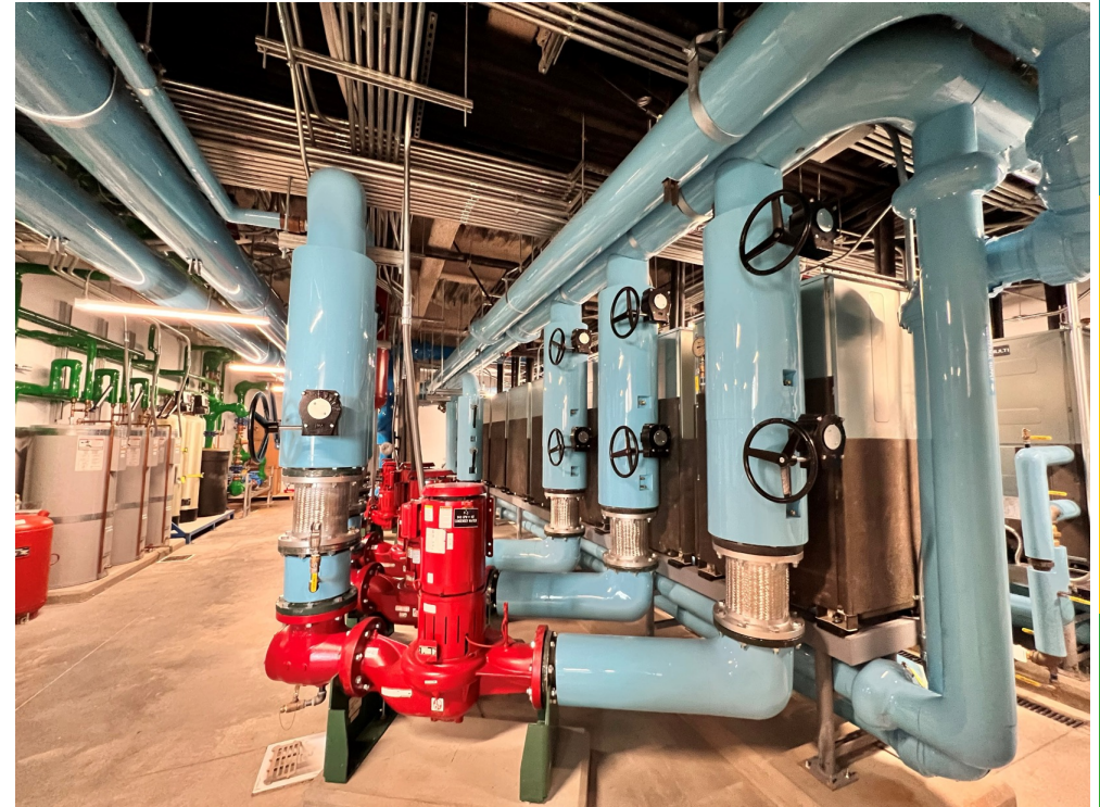
Geothermal heating and cooling system at the University of Utah. Photo courtesy University of Utah.
